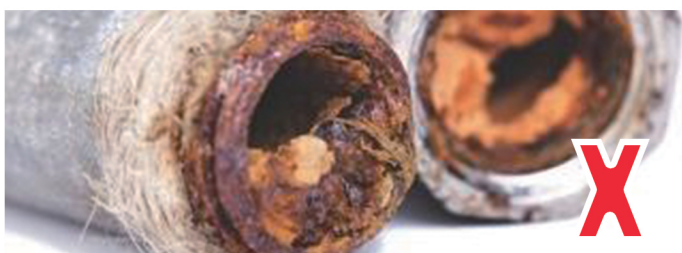
Water pipes WITHOUT help of Crystphos®
